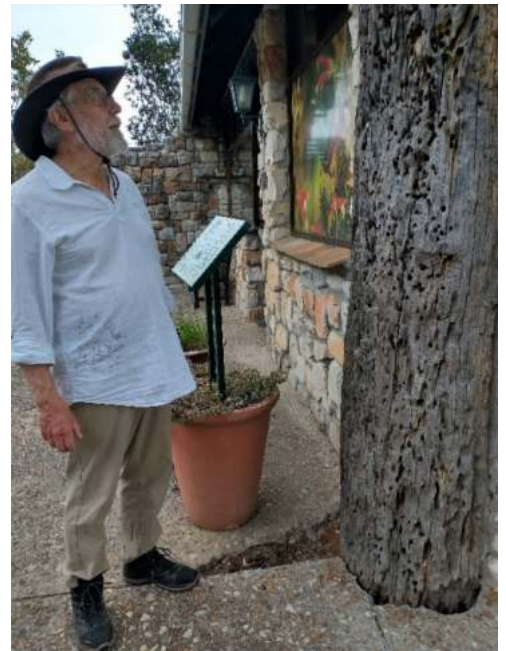
Looking at carpenter bees nest holes in a pillar.
